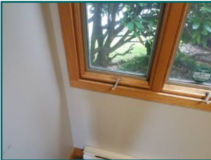
Damaged window crank at rear right corner office
