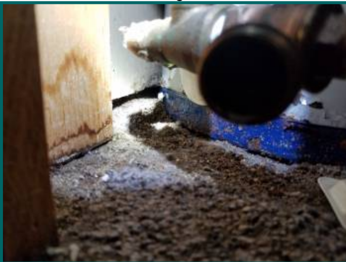
Wet/damp sand around water heater appears to be from condensate
