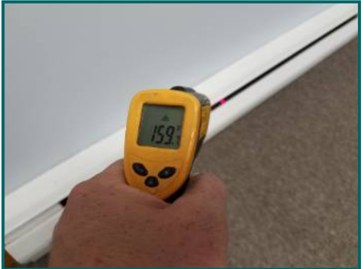
First floor electric baseboard heat working
