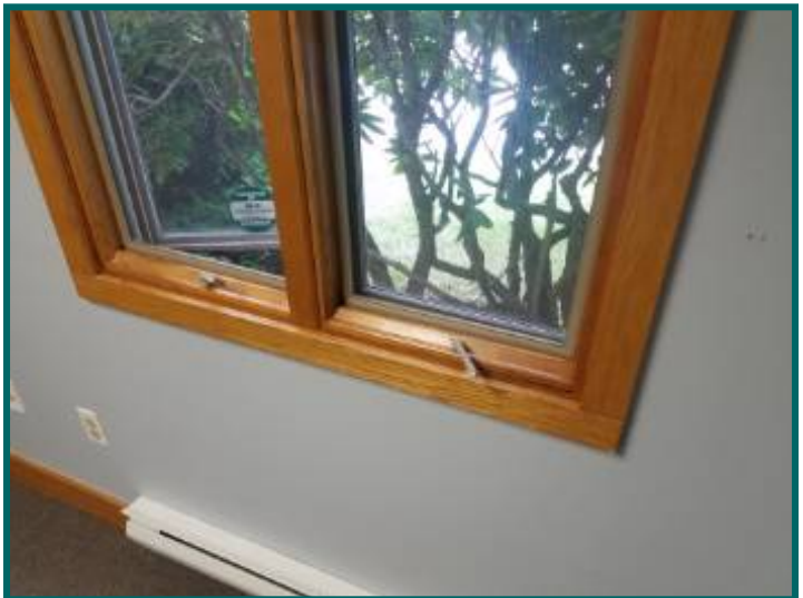
Damaged window crank and heavily corroded crank arm at rear left corner office
