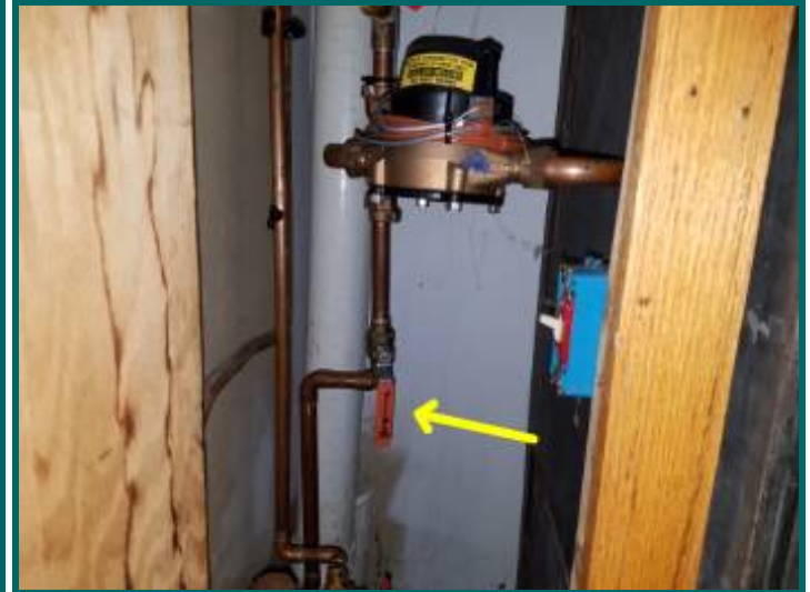
Main water shut off valve is located at water meter
