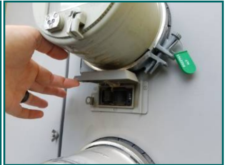
200 amp main disconnect at exterior meter
