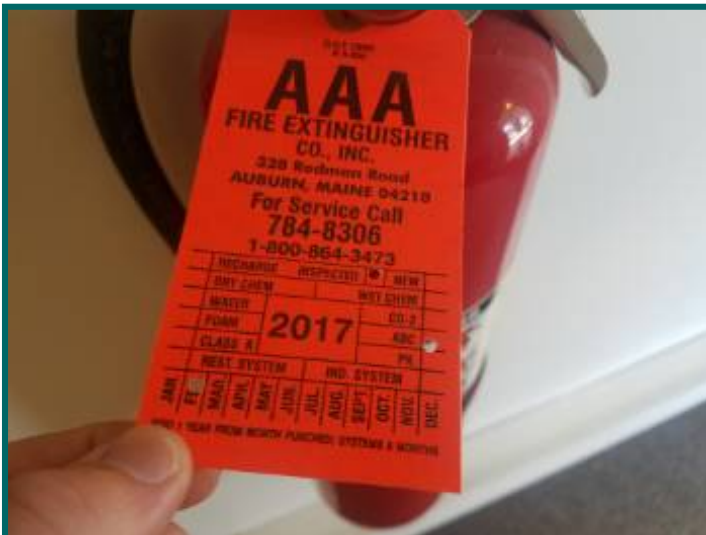
Fire extinguisher tags are expired, dated 2017
