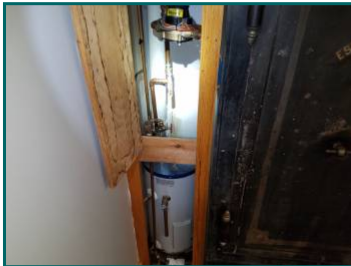
Main drain line termination behind water heater
