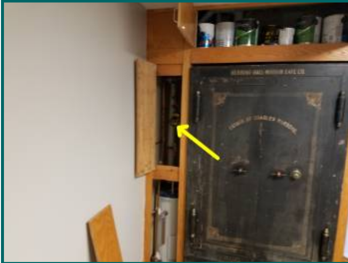
Water meter and shut off valve location
