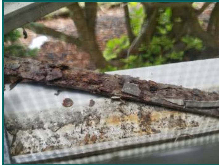
Heavy corrosion on crank arm
