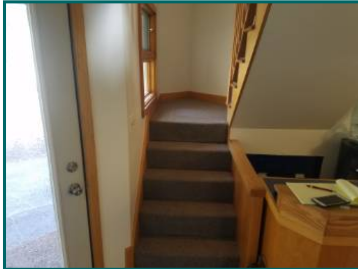
Missing hand rail at first floor
