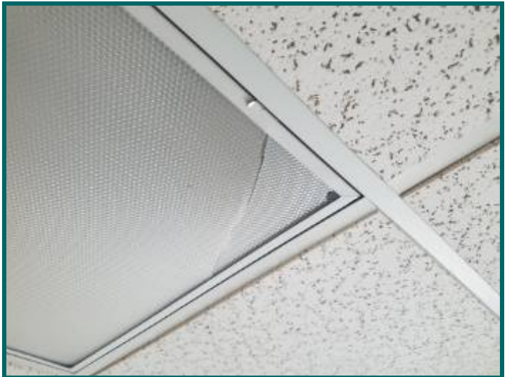
Damaged/cracked lense at first floor hall
