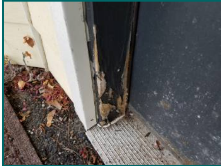
Peeling paint at front entry
