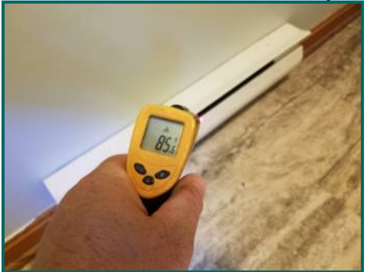
Electric baseboard heater not working at second floor bathroom, may be too hot to test
