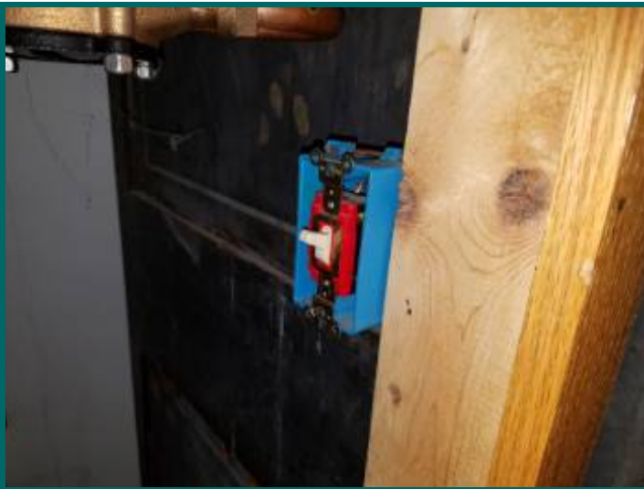
Plate cover missing above water heater
