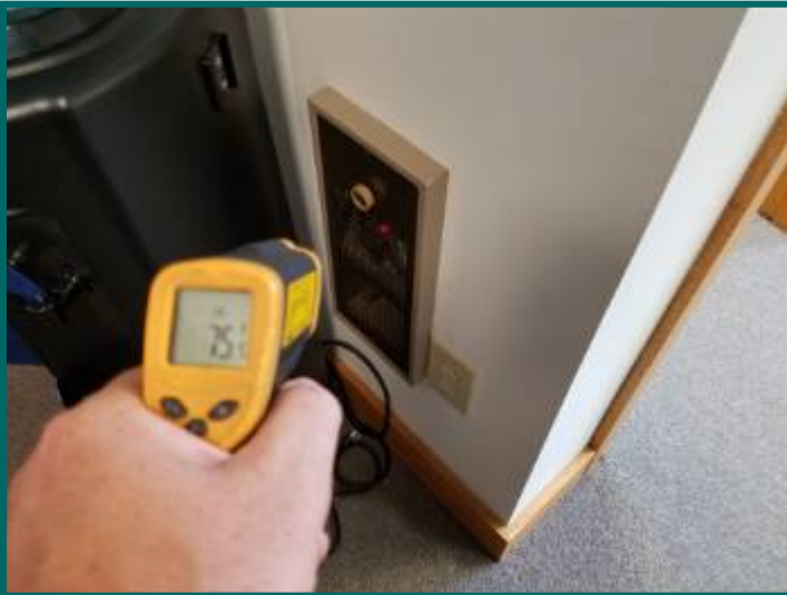
Electric wall heater not working at entry desk area
