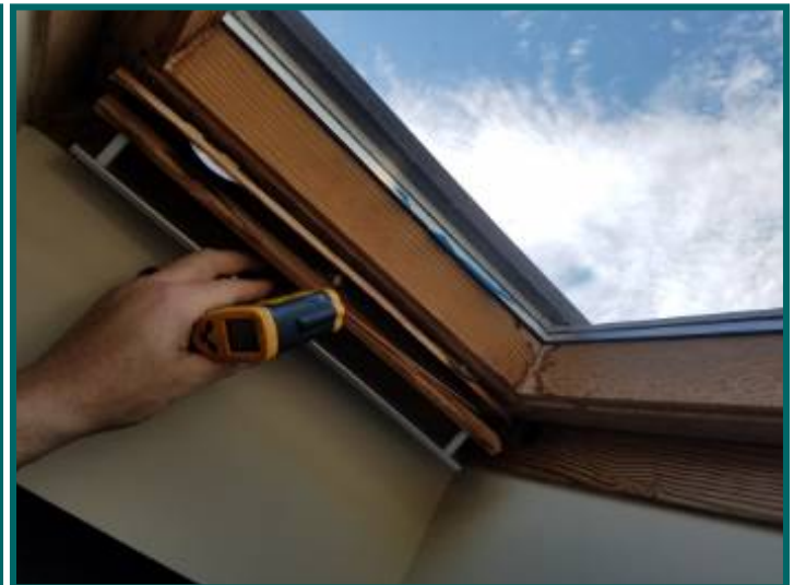
Damaged skylight trim at front
