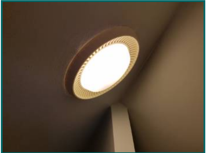
Bath fan not working
