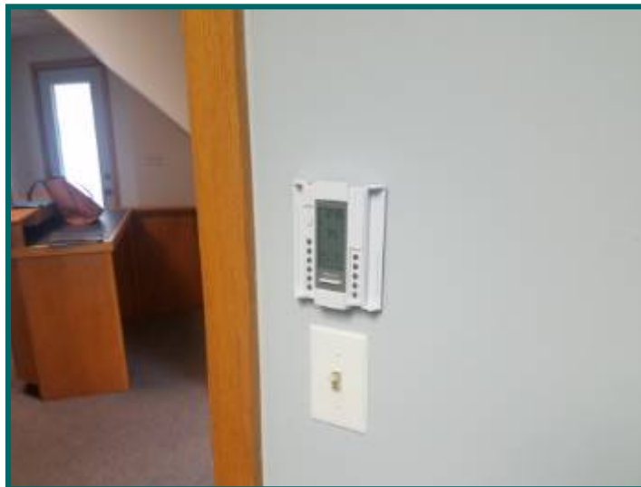
Individual electric heater thermostats
