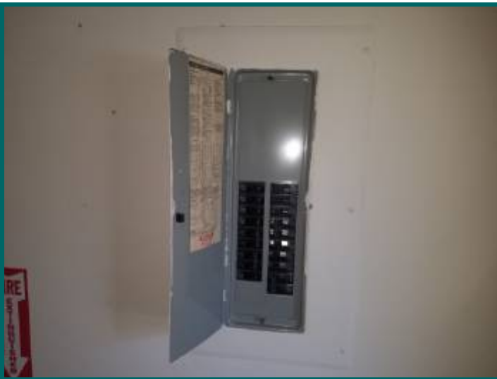
Main panel at entry area
