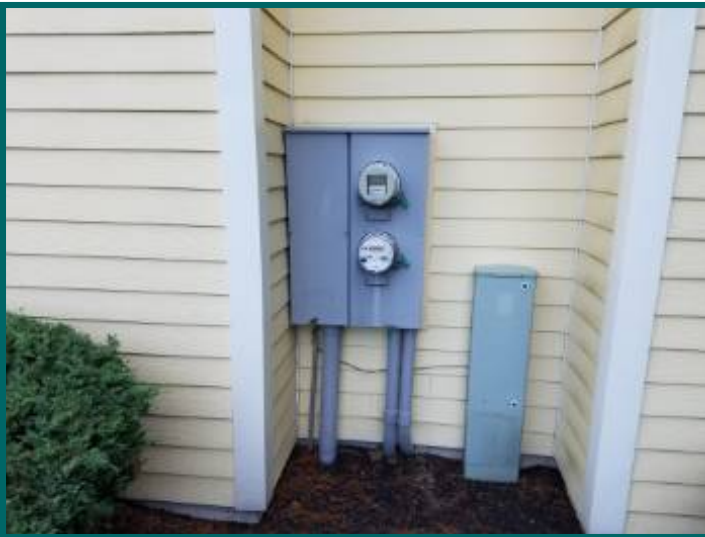
Common meter bank at front, individual meters and breakers are not labeled
