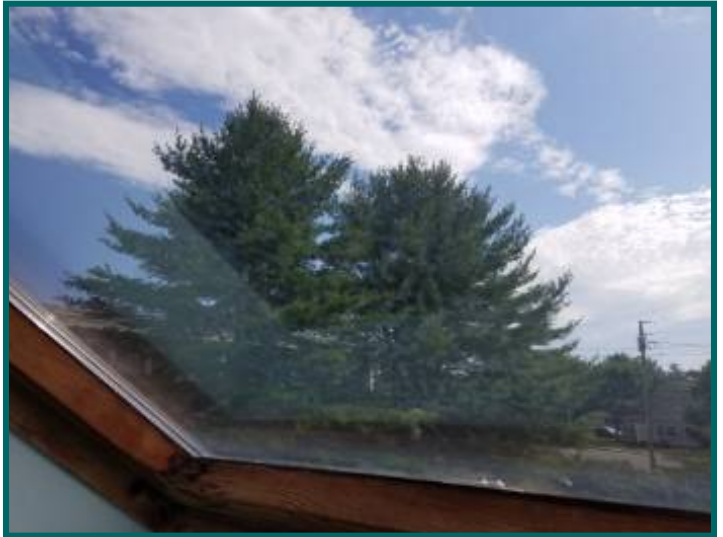
Fogged glass at rear
