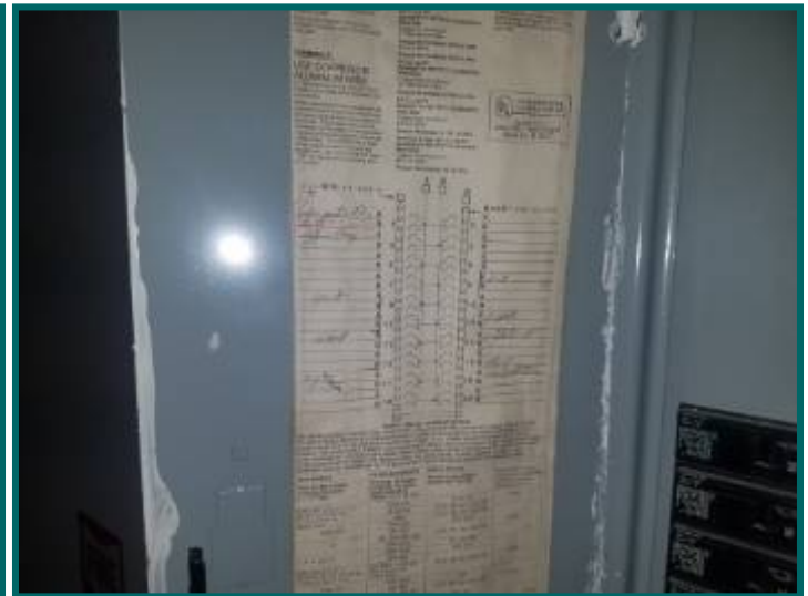
Breakers are not fully labeled
