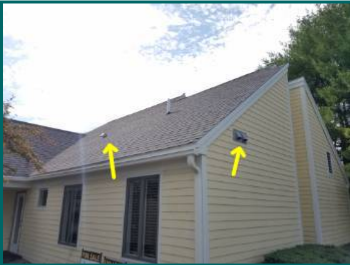
3 exterior terminations, bath fan termination could not be identified
