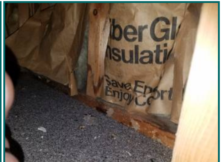
Minor staining on framing below front entry stairs
