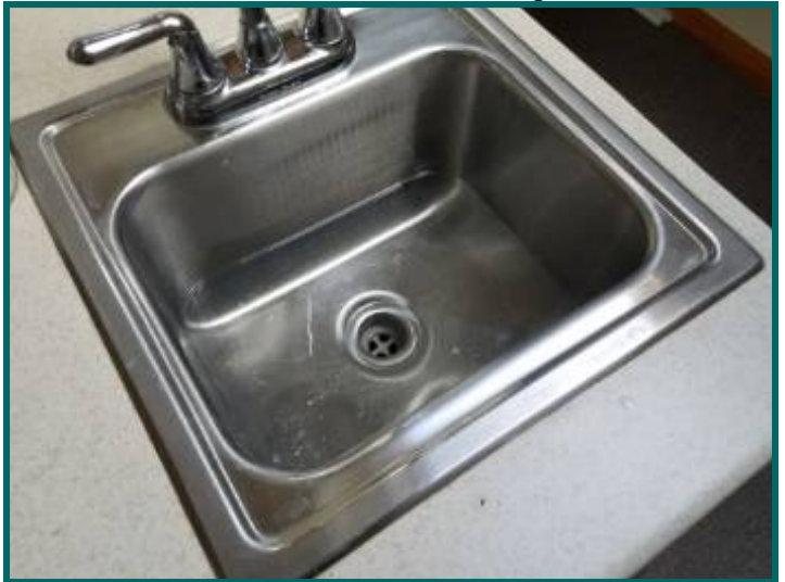
Slow drain at sink, gargling and bubbling, may be venting related
