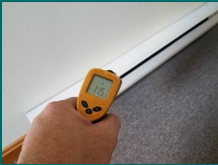
Second floor electric heat
