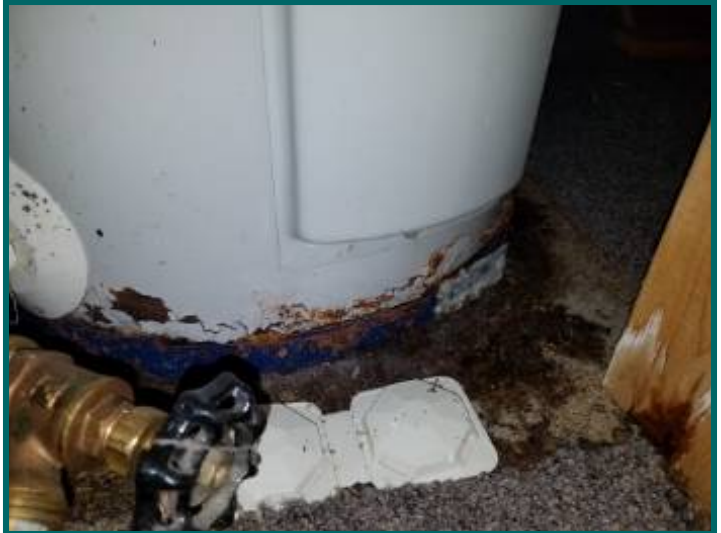
Corrosion on cabinet.
