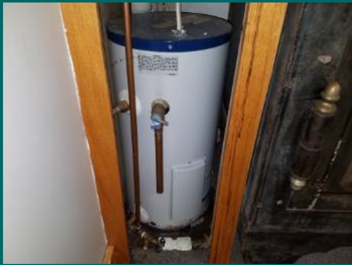
Electric water heater below water meter, 35 years old, 12 gallons
