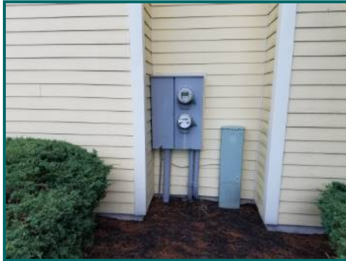
Main service cable entrance
