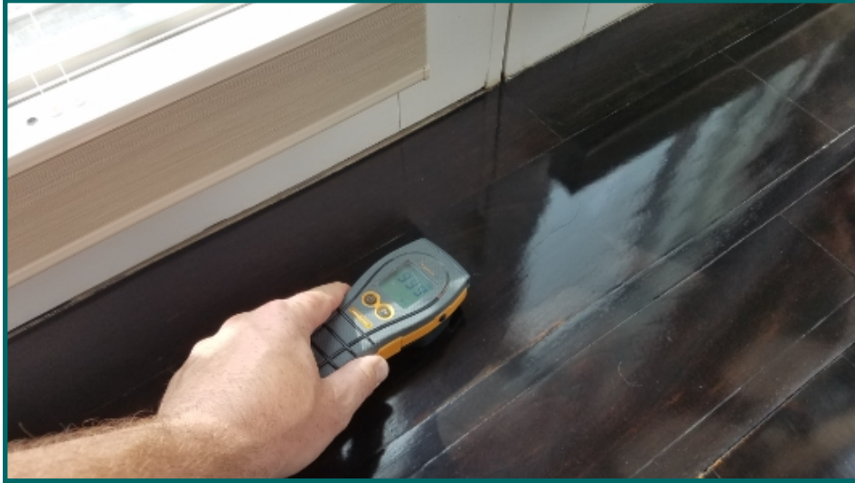
Elevated moisture levels at living room doors
