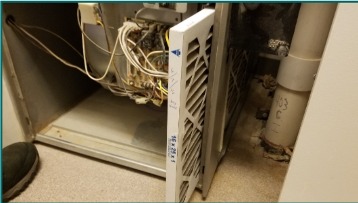
First floor air handler filter
