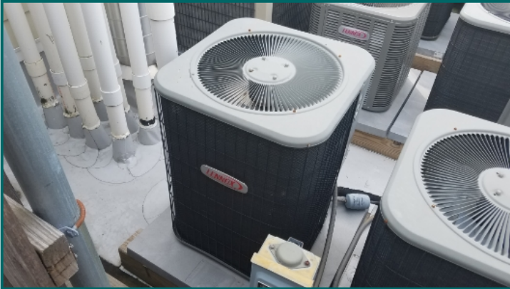
First floor AC
