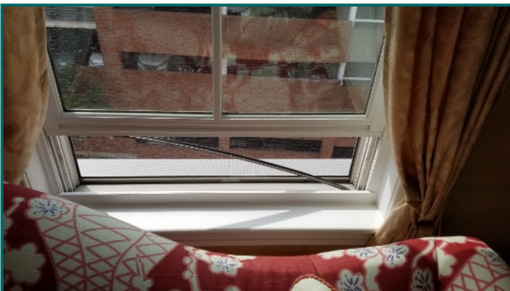
Damaged weather stripping at master bedroom
