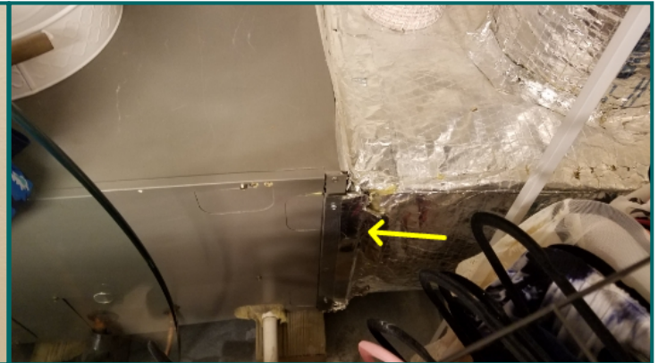
Second floor air handler filter
