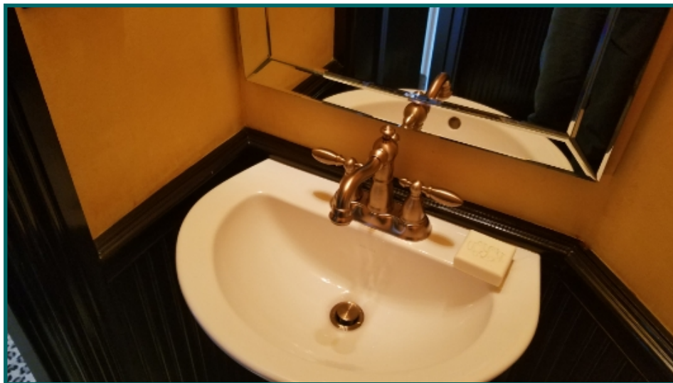
Stopper damaged at hall bathroom
