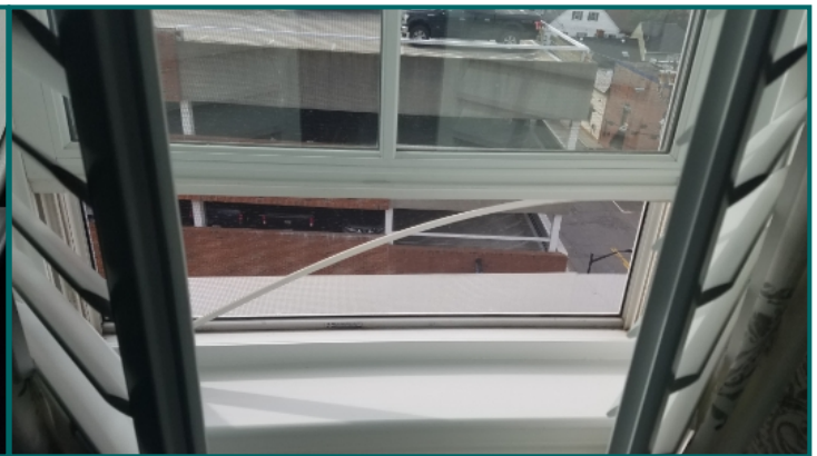
Damaged weather stripping at middle bedroom
