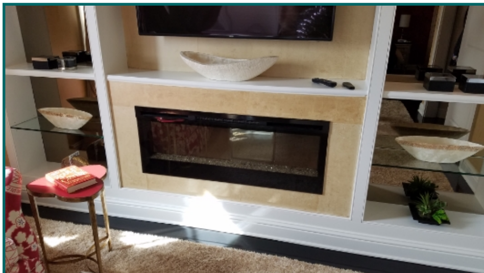
Built in electric fireplaces did not operate when tested.
