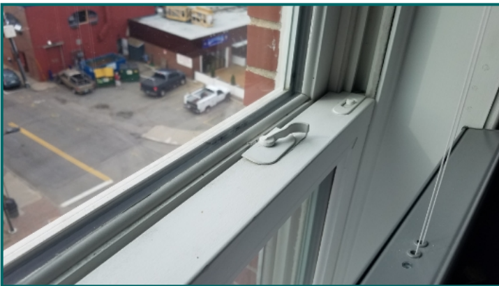
Broken lock at kitchen area
