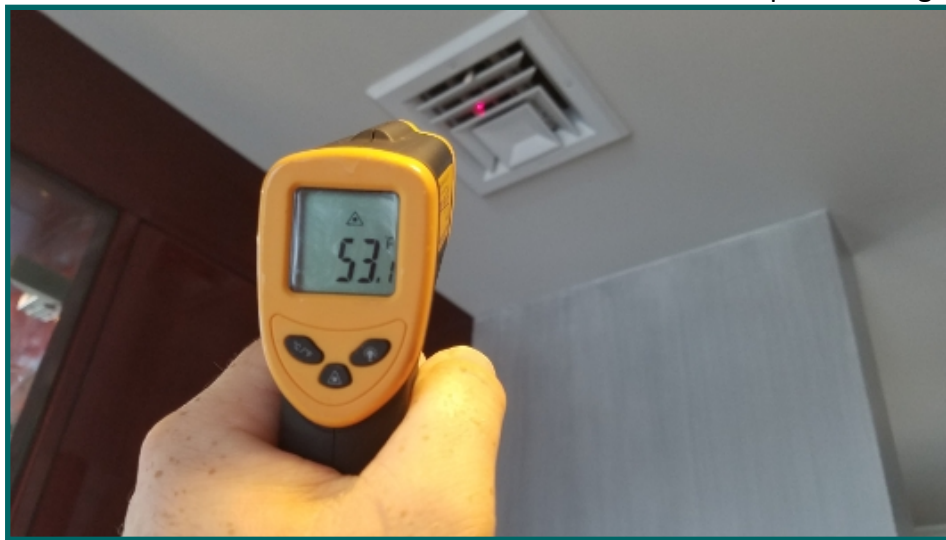
Air blowing cold at first floor
