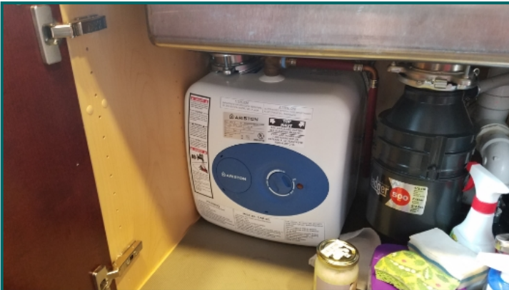
5 gallon electric water heater servicing kitchen sink
