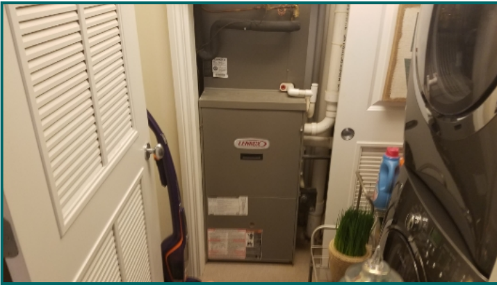
First floor furnace
