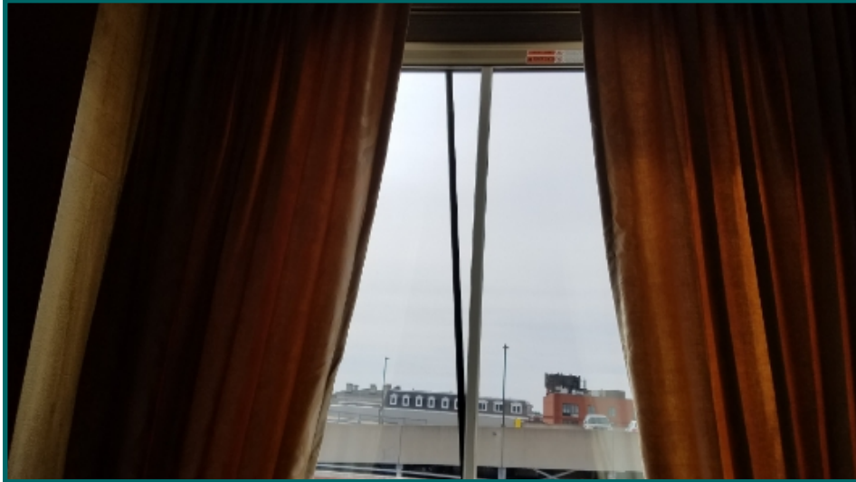
Damaged gasket at master bedroom
