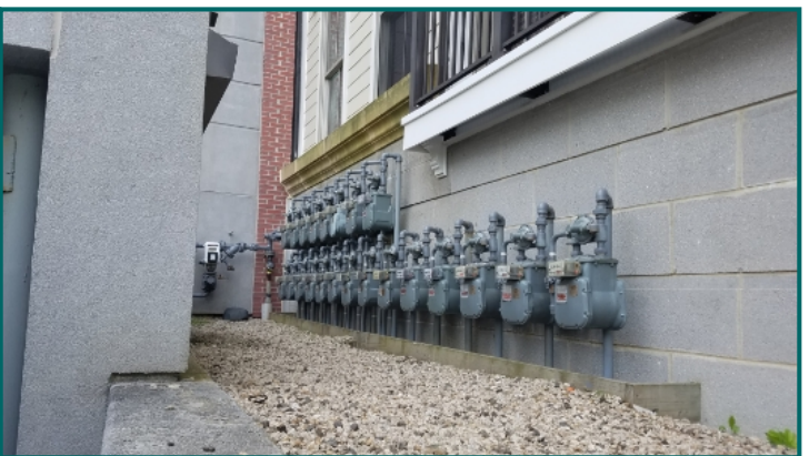
gas meter bank at rear of building
