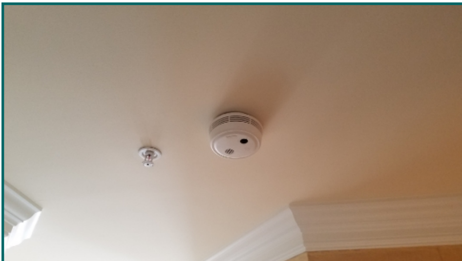
Smoke detectors not tested.
