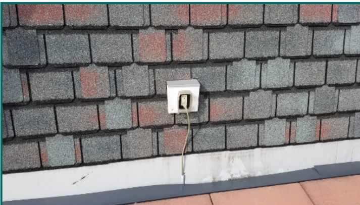
Missing weather proof outlet cover at upper deck
