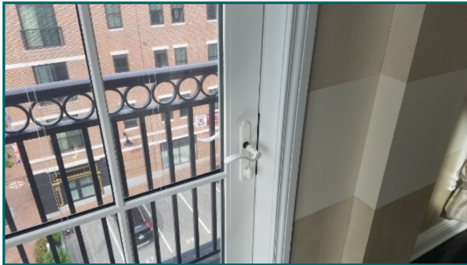
Loose hardware at living room area
